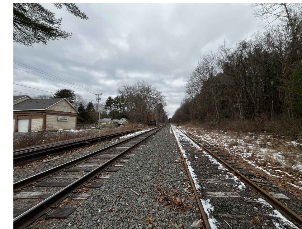
APPROXIMATELY 0.85 MILES OF RAILROAD SIDING ALONG VAN DEUSENVILLE ROAD, GREAT BARRINGTON, NEAR REACH 8
